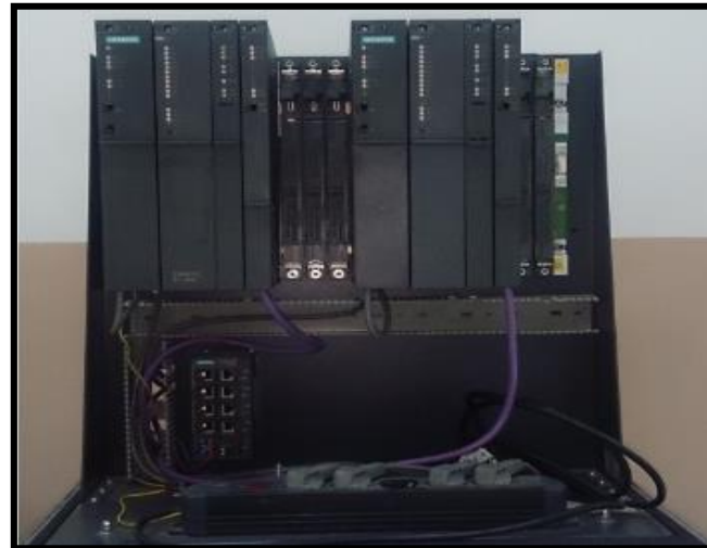
SIMATIC PCS-7 CONTROLLER (S7-400 PLC BASED HARDWARE)
